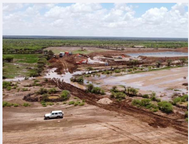
Aerial footage of the construction at the Wado-Makahiil dam, located in Maroodi-Jeex, Somaliland
