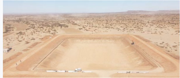
Aerial footage of the construction of Ijaara Hafir Dam (132mX92mX6m) with storage capacity 57,863.00 cubic meters. This dam is located in the South East region of Gabiley, Somaliland.
